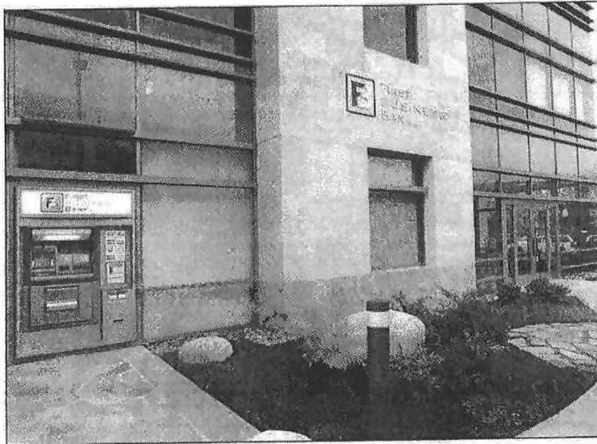
Improvements to First Business Bank, located in Del Mar, include a new exterior ATM installation and suite entry.
